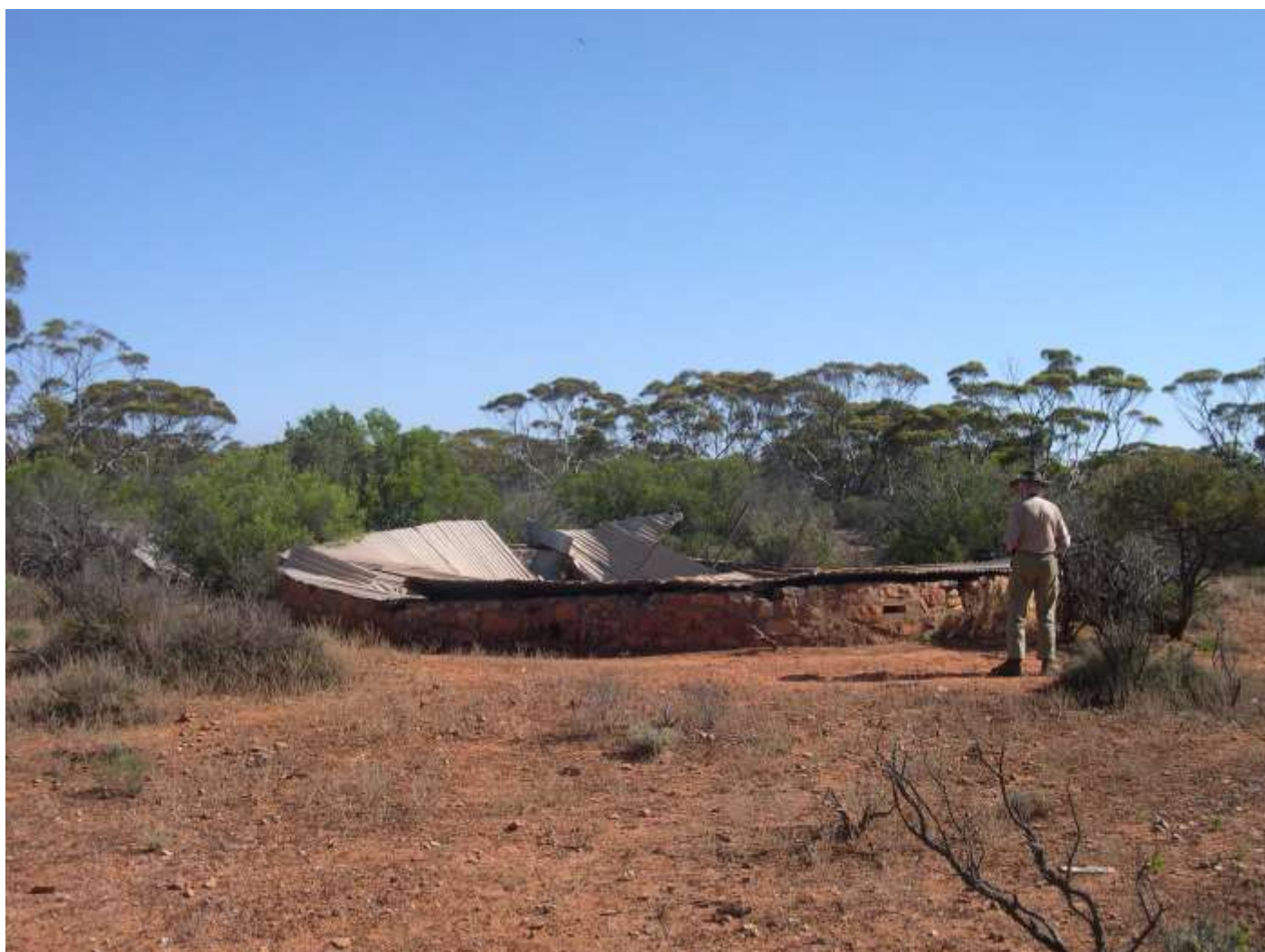
The underground tank on Munyaroo Conservation Reserve on Eyre Peninsula . The Author is shown inspecting the tank.
