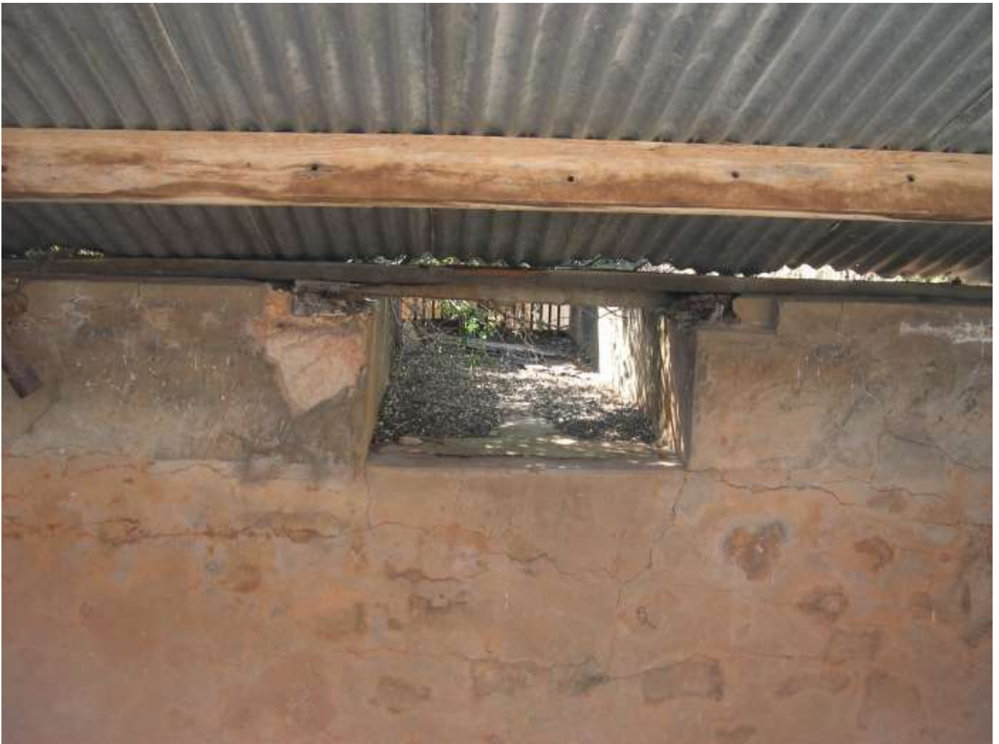
The outlet from the smaller tank to the main tank.
